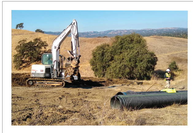
Bayberry Construction – After the backhoe resculpted the gully to make it wider and shallower, the pipe was placed in it and the gully was filled in.
